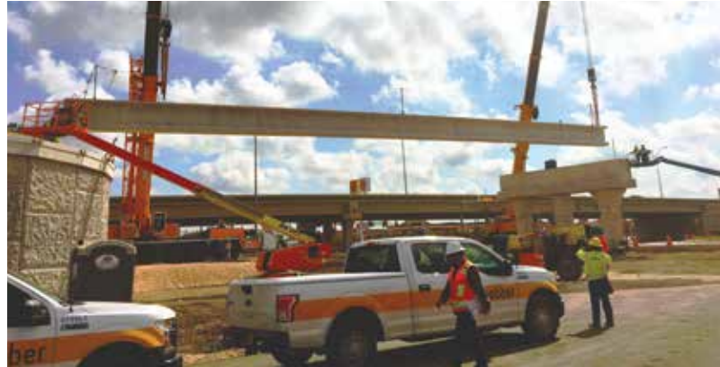
We set the first concrete girders in our Central Texas region last week! These TX 62 concrete girders span at a length of about 137 ft and are located in San Antonio, TX on our Loop 1604 project with Marbach Rd.
